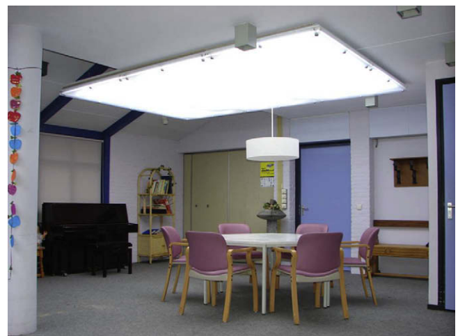
Fig. 2. Experimental luminaire as installed in the day care centre.
